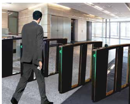
Turnstile Access System
